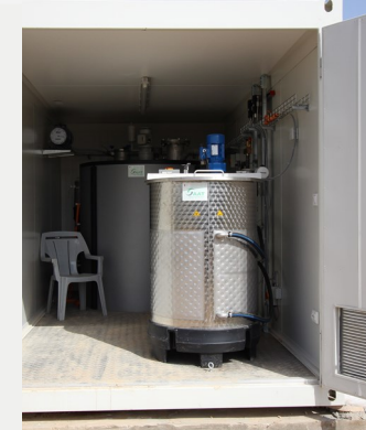
Buffer Tank (front) and Digester (back)
